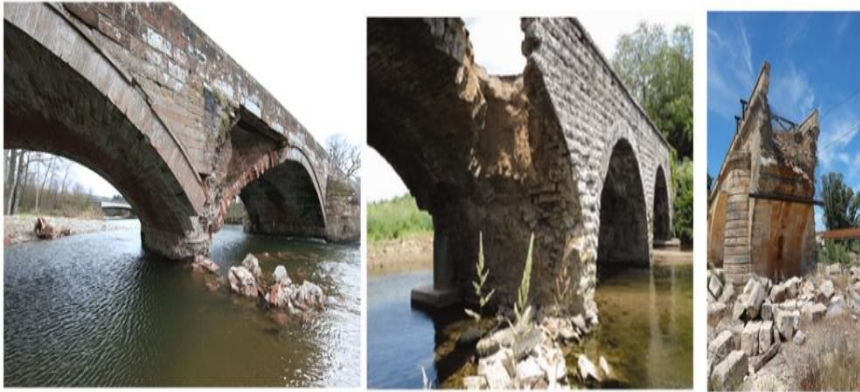
Figure 3 Examples of damaged stone bridges
