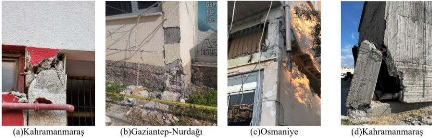
Fig. 17 Short column damages
