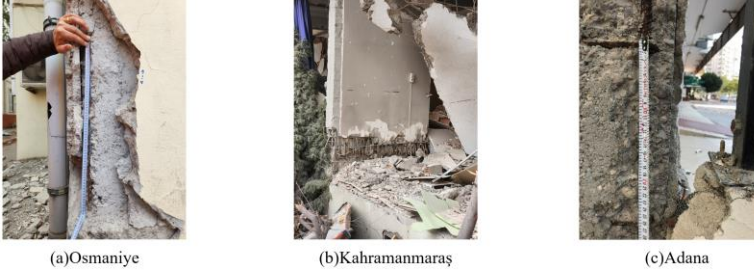
Fig. 21 Inadequate stirrup spacing
