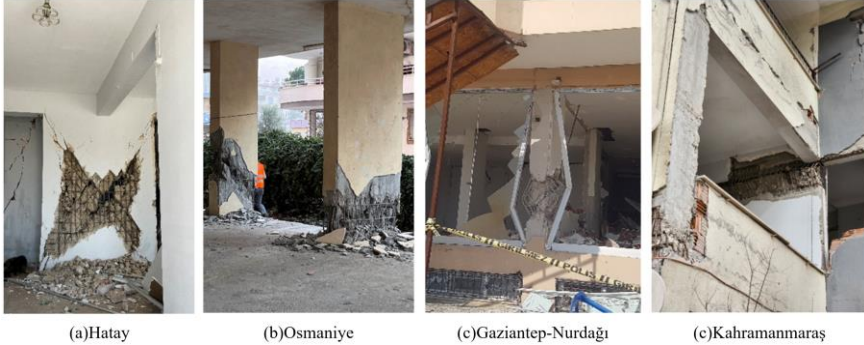
Fig. 14 Columns and shear walls damages
