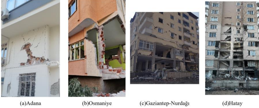
Fig. 12 Observations of infill wall damages
