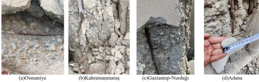
Fig. 24 Damage due to insufficient concrete strength and improper aggregate usage
