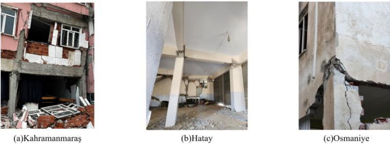
Fig. 22 Column-beam joint damages
