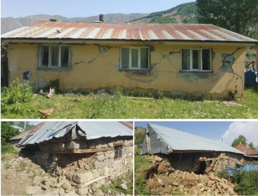
Figure 9. Examples of masonry structures damaged in the 2020 Bingöl-Karlıova Earthquake
