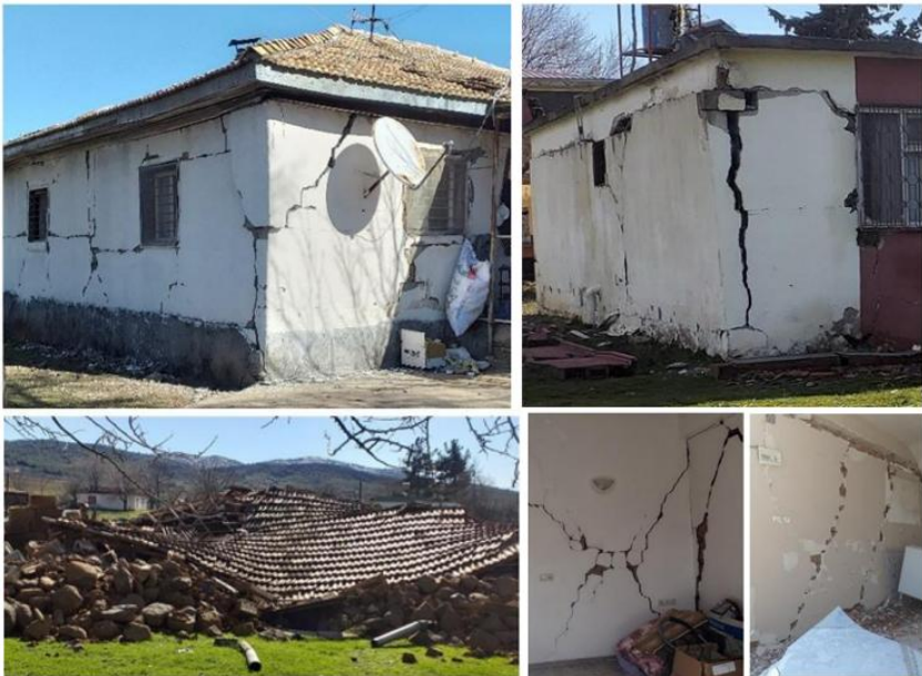
Figure 8. Examples of masonry structures damaged in the February 6 Pazarcık Earthquake
