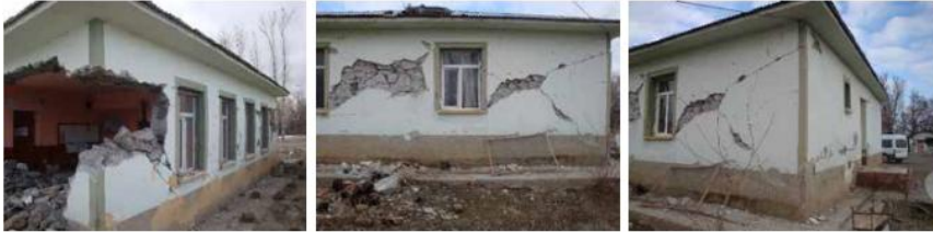
Figure 7. Examples of masonry structures damaged in the 2011 Van Earthquake
