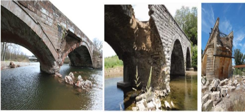
Figure 3 Examples of damaged stone bridges
