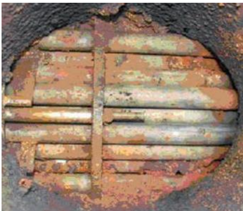
Figure 10: A heat exchanger exposed to corrosion contamination
