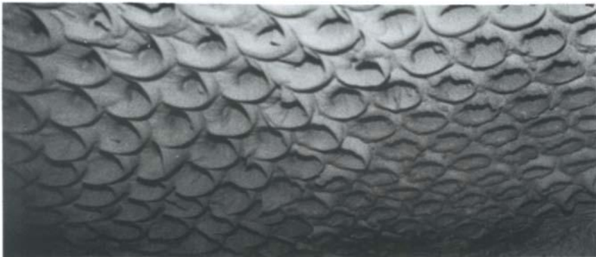
Figure 3: The fouled inner surface of a shell-and-tube boiler
